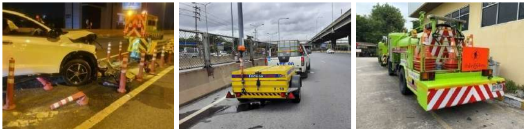
Actions taken to reduce severity of accidents: installments of crash cushions and truck mounted attenuators
